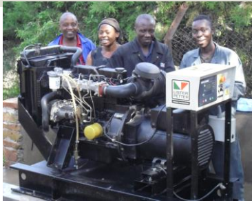
Electricians Stephen, Lavinia, Philemon and their apprentice with the new emergency diesel generator set awaiting the now completed housing (inset)
